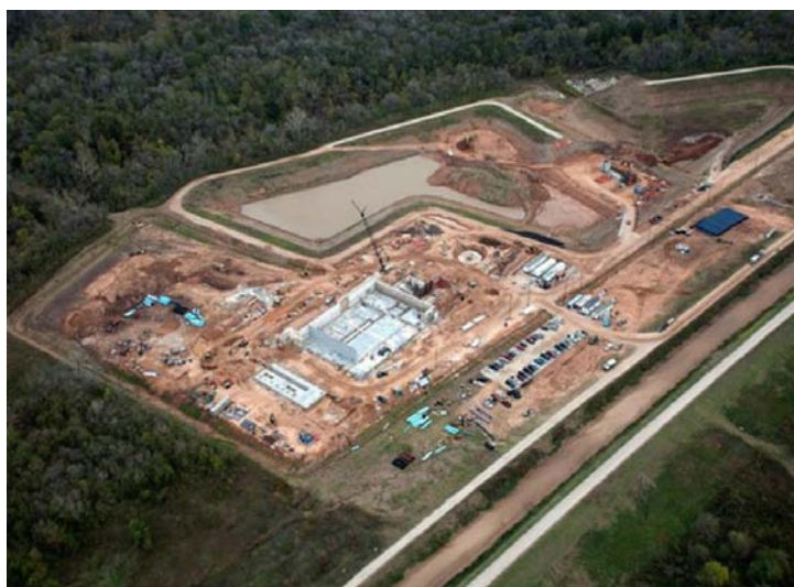
Aerial Photo 727.520.8881 www.aerophoto.com Missouri City Surface Water Treatment Plant Image # 101130 6068 Date 11.30.10
